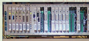
NEC ISC-303 Digital Telephone System
